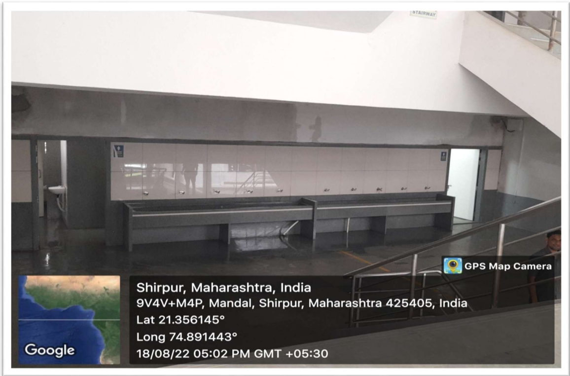
Infrastructure upgradation: Lavatories and Drinking water facility
